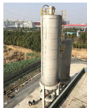
存储料仓 Storage Silo
